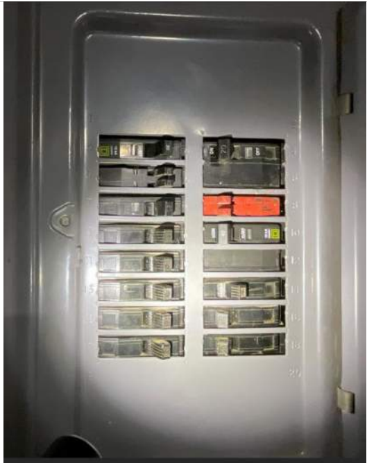
Photo #3: Load Center - Basement
