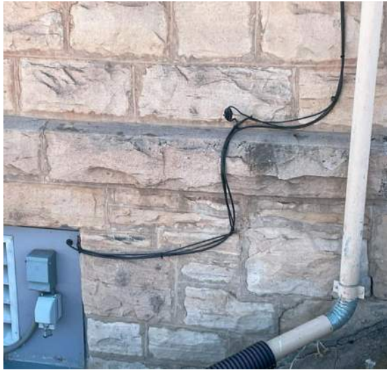
Photo #16: Co-axial cable entering the building
