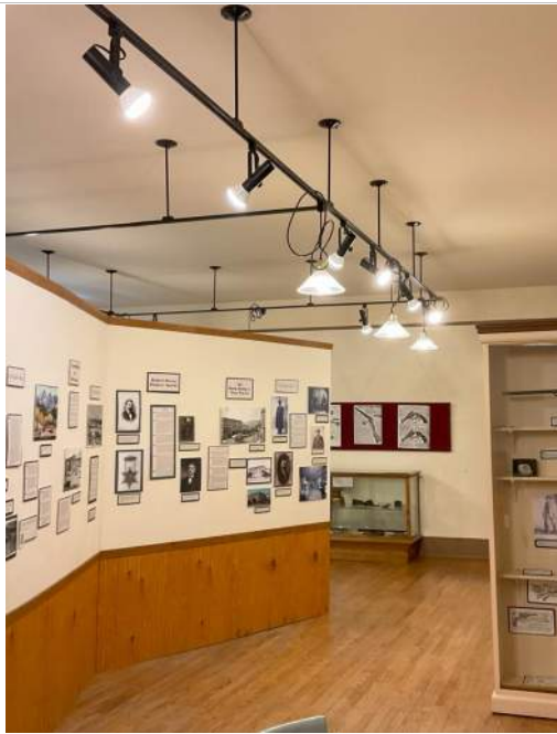
Photo #7: Track lighting in gallery spaces with LED lamps
