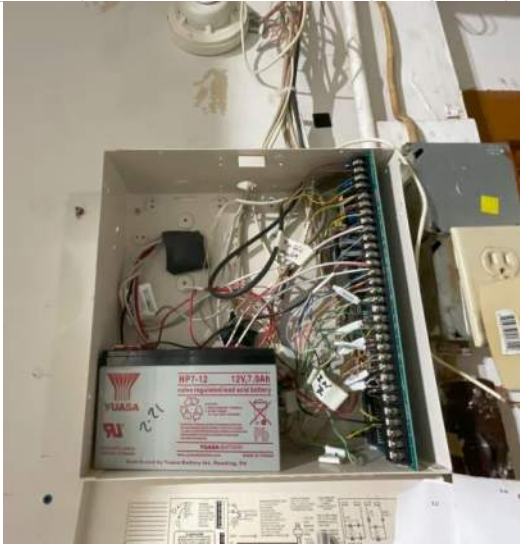
Photo #19: NetworX Security Cabinet in basement
