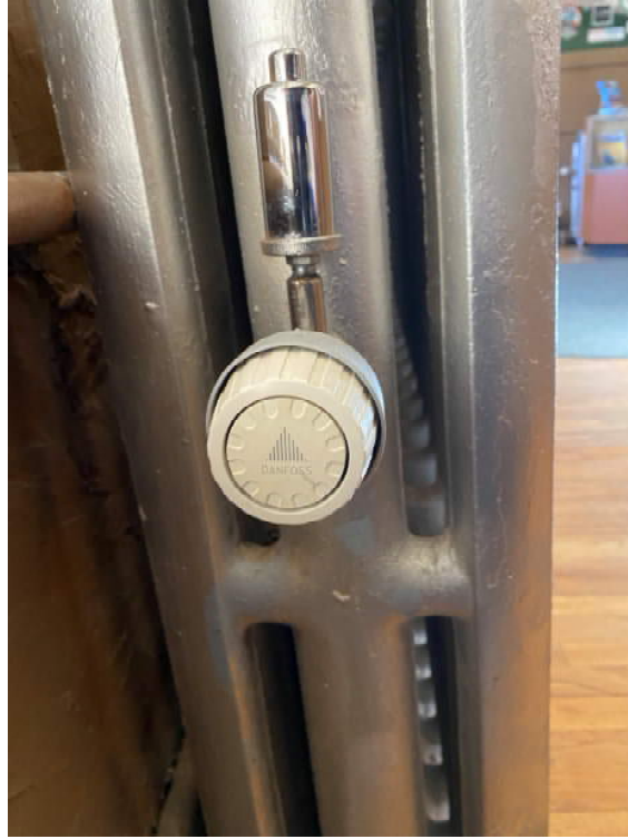
Typical Danfoss Valve Installed in Radiator Air Aspirator
