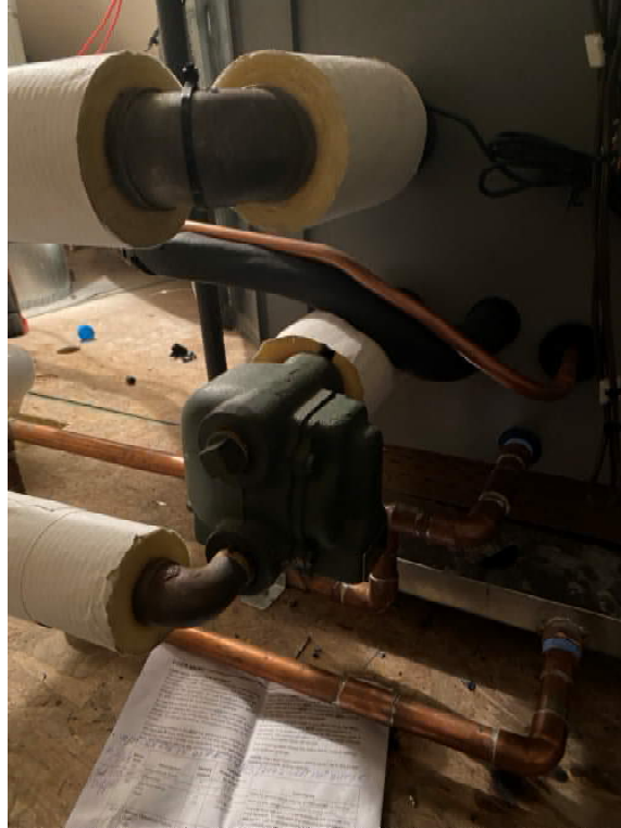
STEAM Connection to Attic Fan Coil Unit
