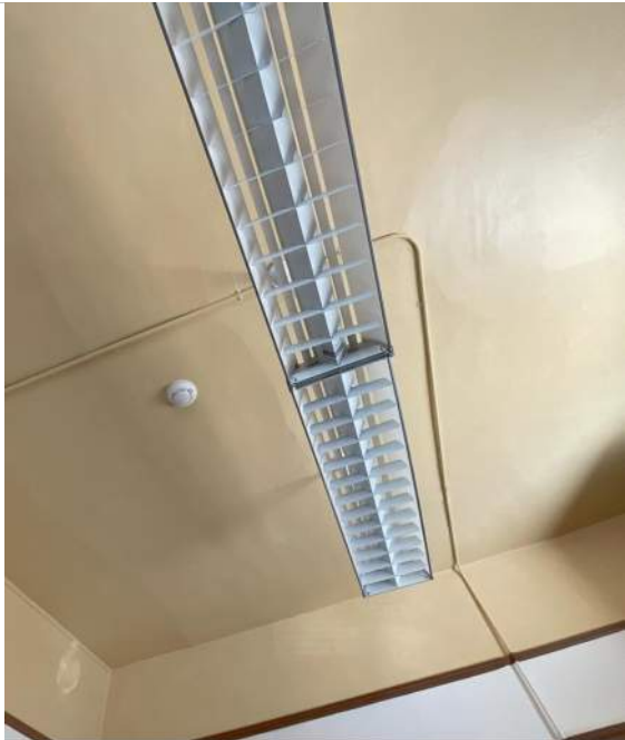
Photo #8: Fluorescent Light fixtures
