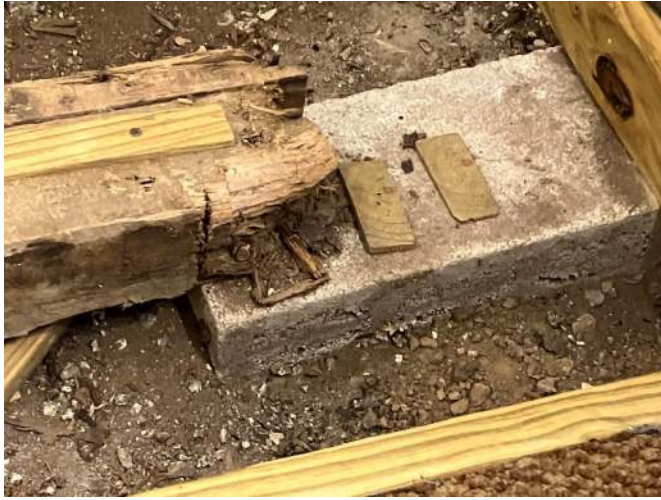
Second Area of Deteriorated Floor
