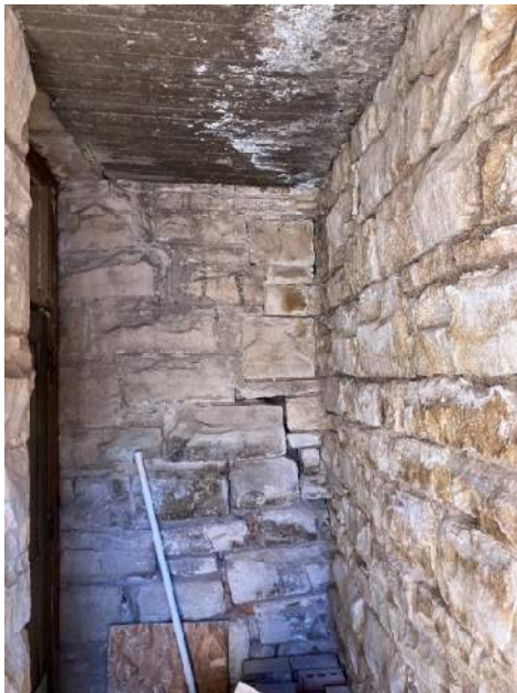
Stairstep Cracking from Movement of Entry Stair
