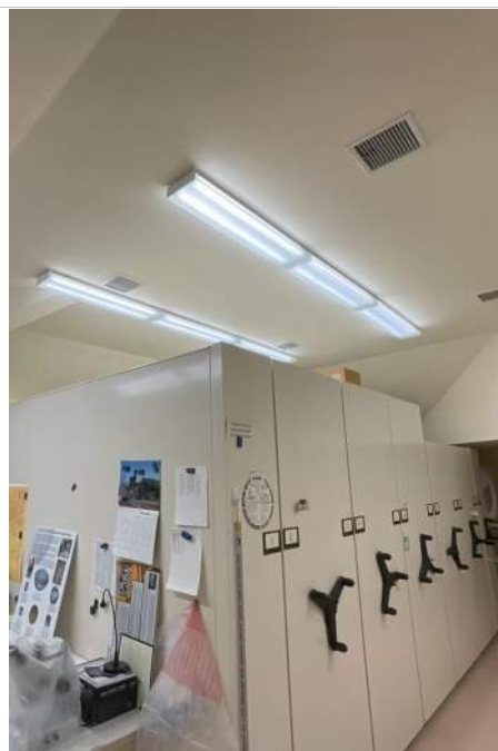
Photo #12: Fluorescent fixtures in attic
