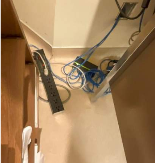
Photo #6: Extension cords in use
