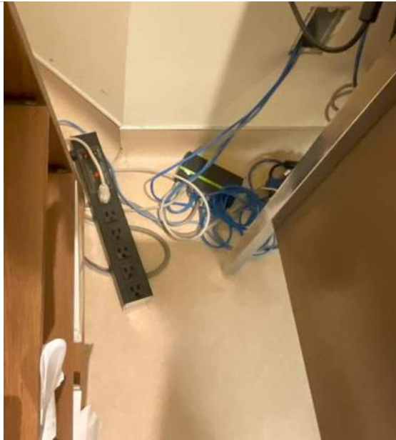
Photo #20: 8-port Network switch in Attic
