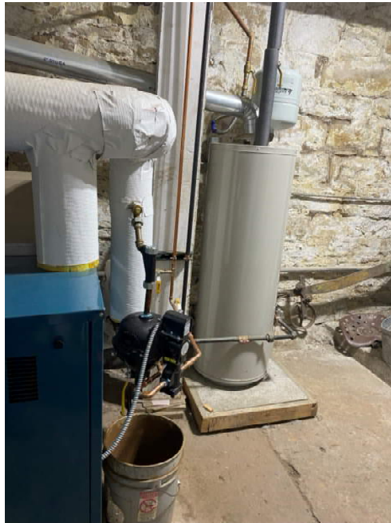
Existing Water Heater in Mechanical room
