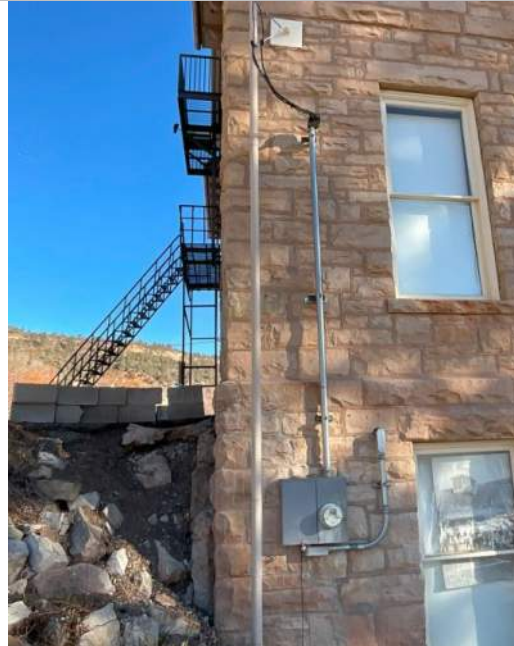
Photo #2: Existing utility meter
