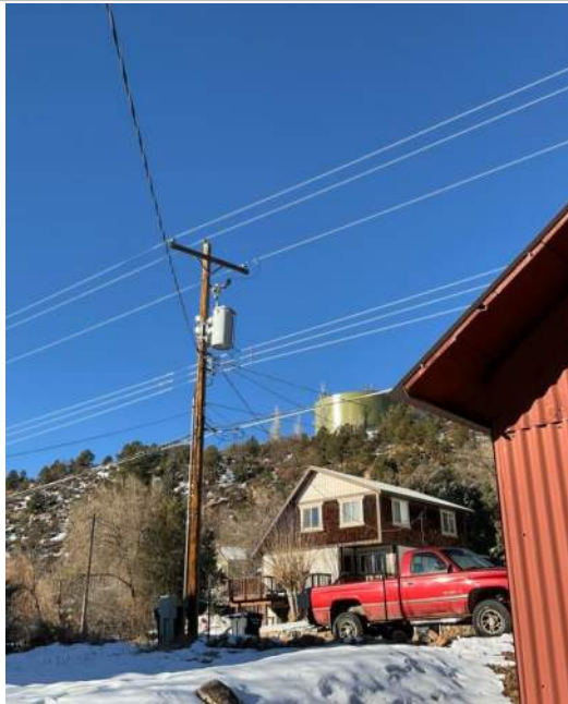
Photo #1: Existing pole-mounted utility transformer
