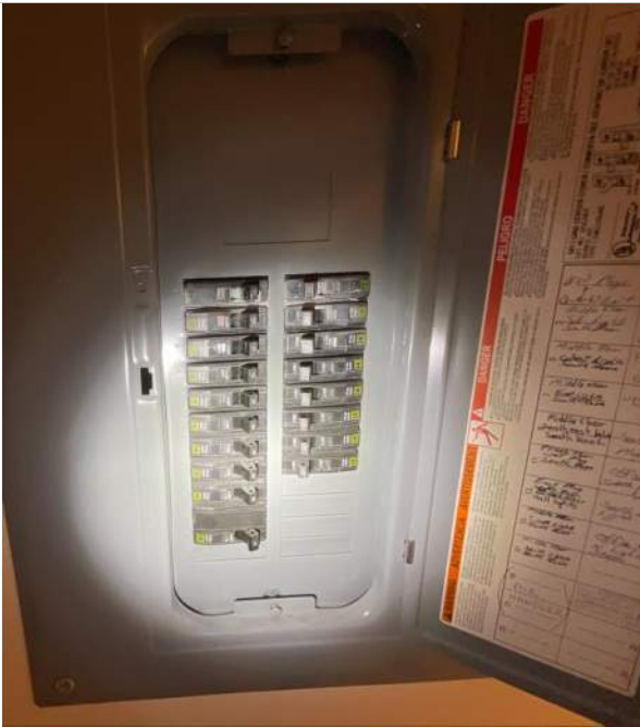
Photo #4: Load Center - Attic
