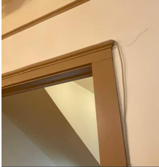
Photo #5: Exposed Cabling around doorway
