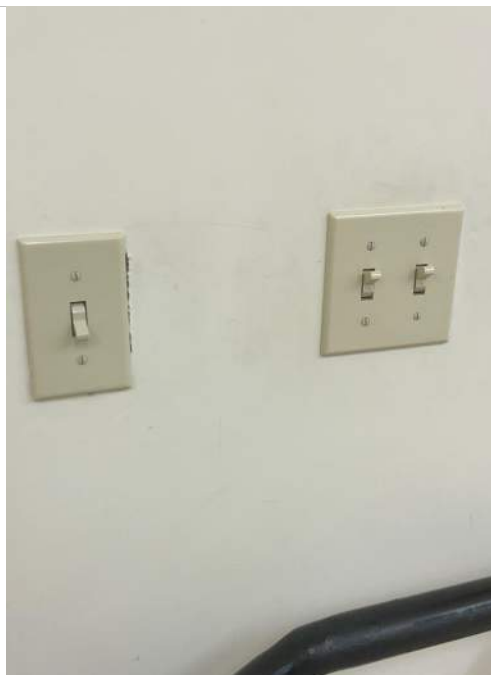
Photo #11: Manual line voltage light switches
