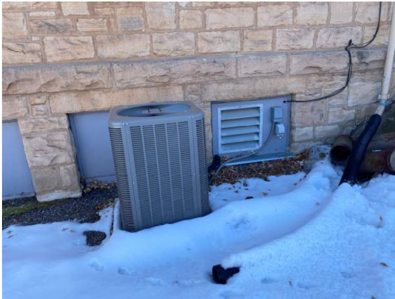
Condensing Unit for Attic Fan Coil Unit and Combustion Air Louver for Boiler and Water Heater
