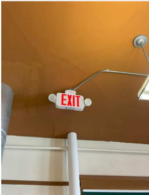
Photo #9: Emergency Lighting/Exit Signs
