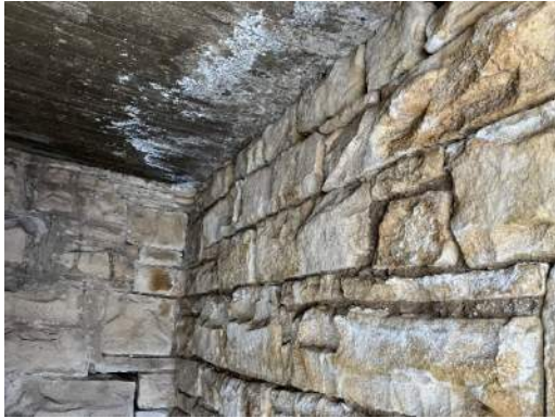
Deterioration at Stone Stair from Water
