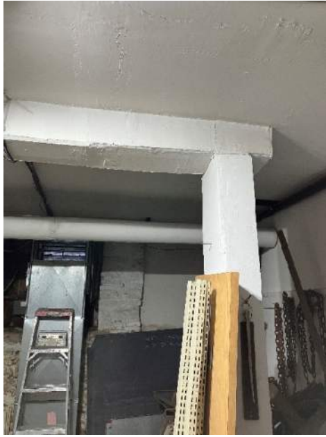
Frames in Boiler Room Supporting Broken Floor Joists
