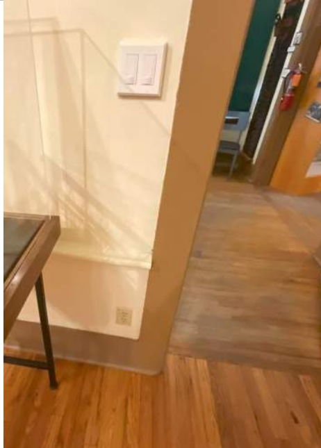
Photo #10: Wall-switch sensors in gallery spaces
