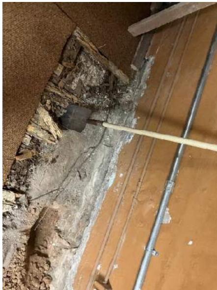
Deteriorated Floor Framing on Sleepers on Grade
