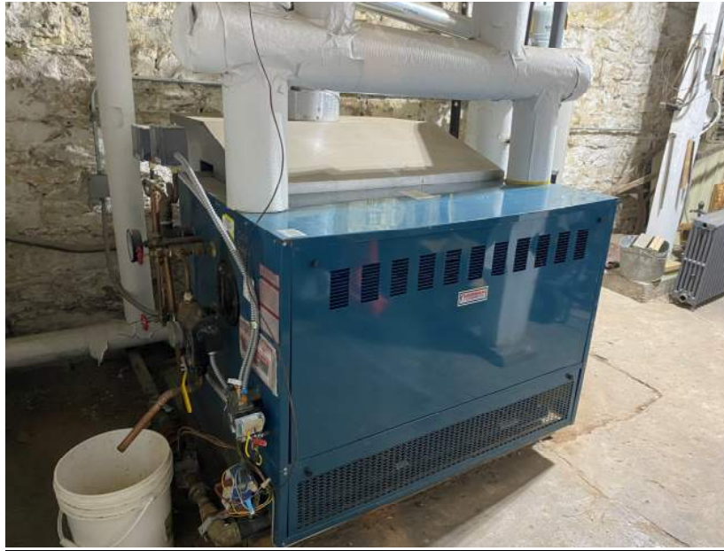
Existing Boiler in Mechanical Room
