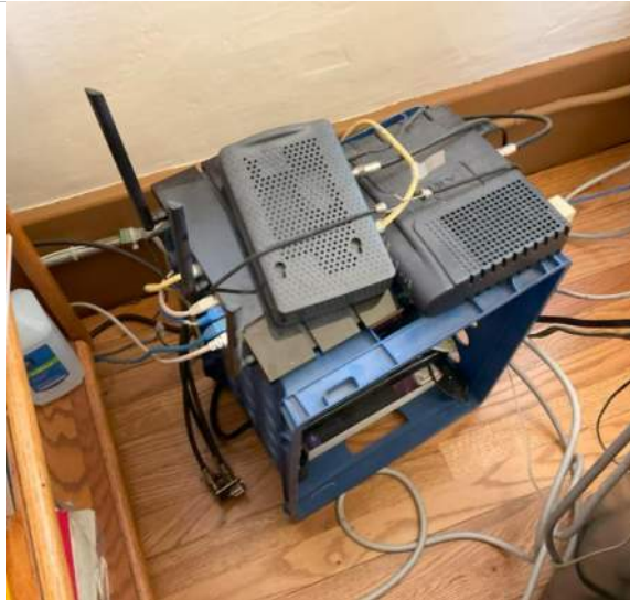
Photo #18: Splitter and modems on first floor
