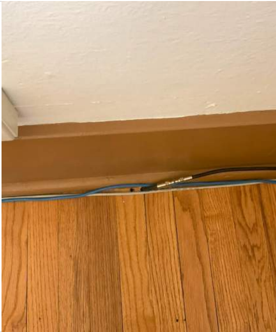
Photo #17: Internet cable routed through floor (from exterior of building to splitter)
